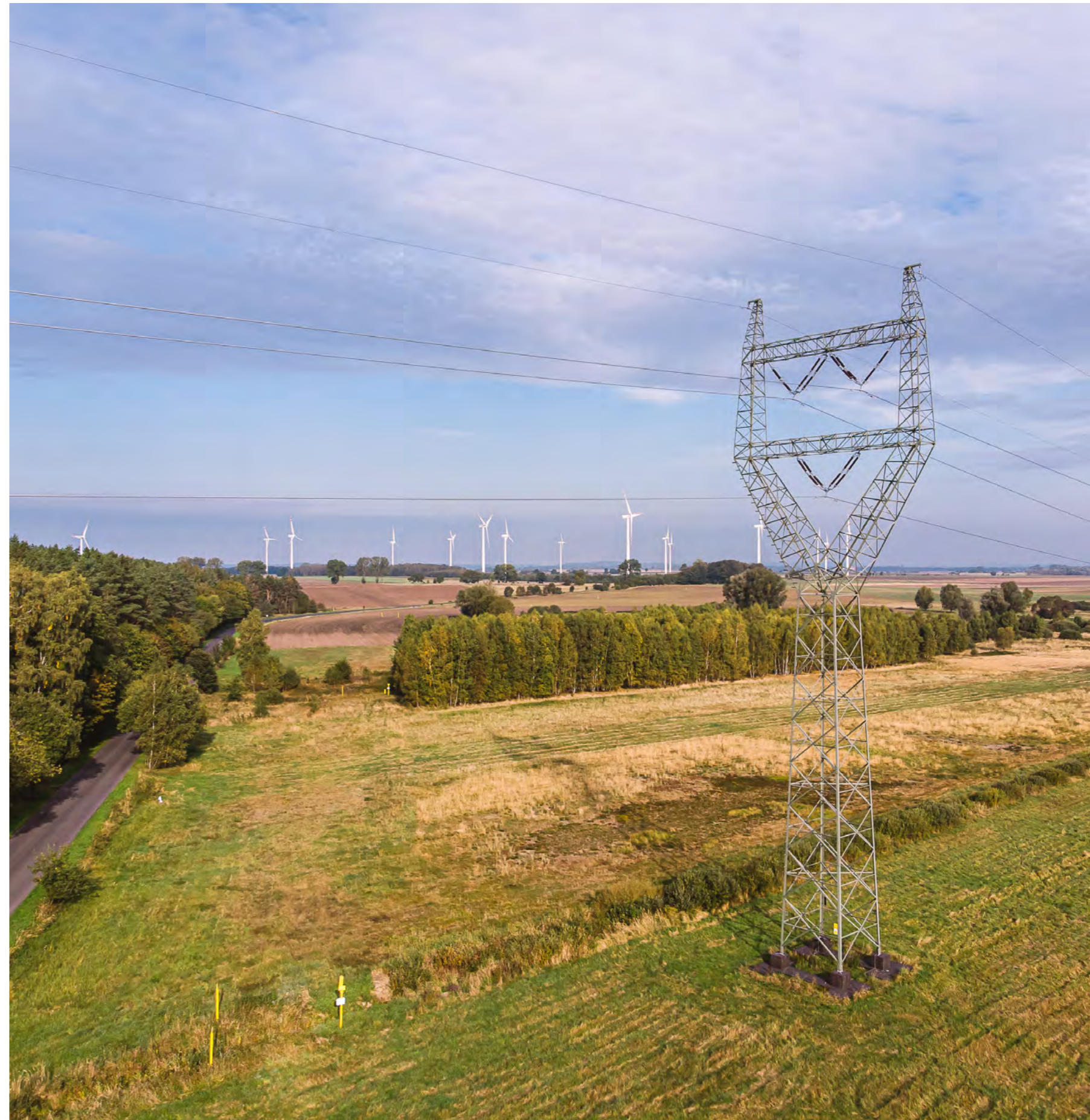
PSE, Linia 220 kV Glinki – Reclaw
